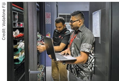
ATH's largest costs of business are in sourcing bandwidth and equipment.
